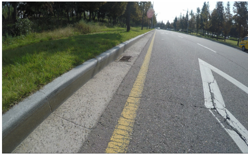
Fig. 11. Damage of Road Marking
