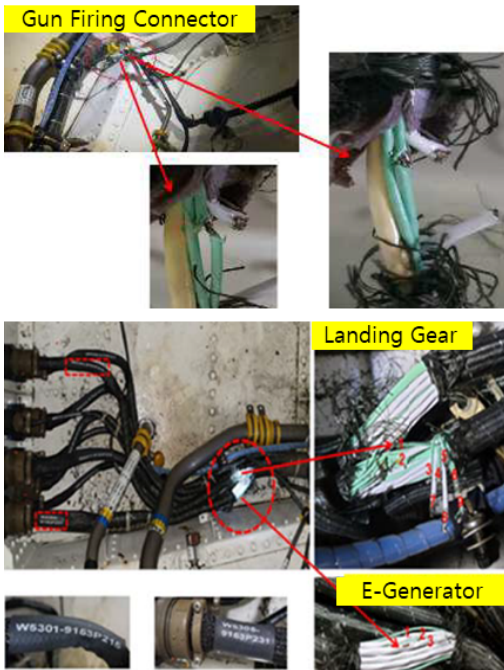
Fig. 4. Wire Harness Defects in Gun Bay
