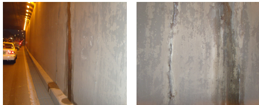
(a) 누수 (a) Water leak (b) 균열 백태 (b) Crack and efflorescence
