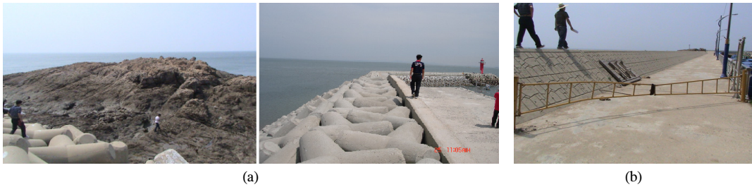
[Fig. 5] Facility for restricted area (a) Omitted installation in hazardous area (b) Ineffective installation
