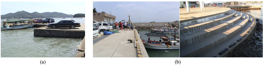
[Fig. 6] Car stopper (a) Omitted installation in hazardous area (b) Improper placement
