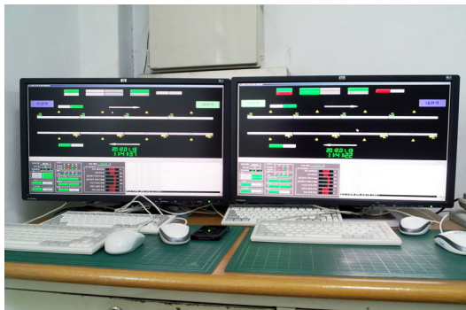
[Fig. 5] Maintenance Monitor of Station Control Unit
