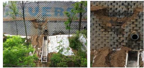
[Fig. 3] Appearance and condition after 1st failure
