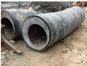
[Fig. 6] Bowed drainpipe(PE double wall pipe)
