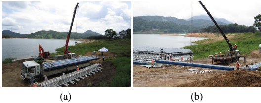
[Fig. 4] Bringing in FRP structure (a) Bringing in material and unloading (b) Unloading buoyancy structure
