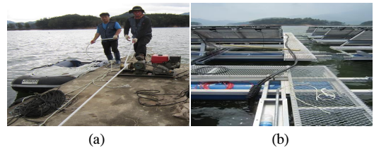
[Fig. 17] Construction of underwater cable (a) Cable installment using winch (b) Underwater cable installment
