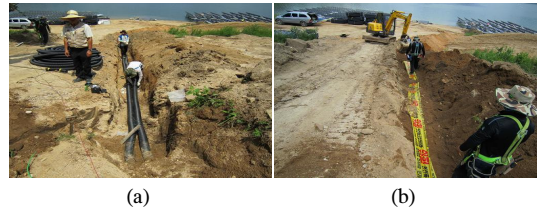
[Fig. 16] Laying of overland portion of underwater cable (a) Pipe routing in available underground area (b) Submersion section in case of rise of water level
