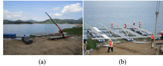
[Fig. 6] FRP structure refloat and launch into water (a) FRP structure refloat (b) Launch into water
