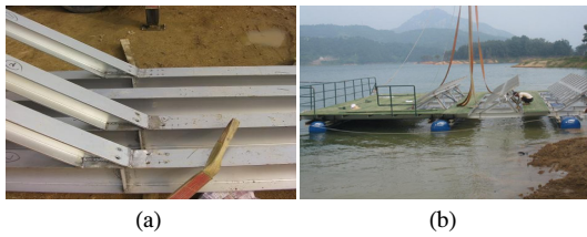
[Fig. 8] Aluminum structure launch into water (a) Structure bolt assembly (b) Launch into water
