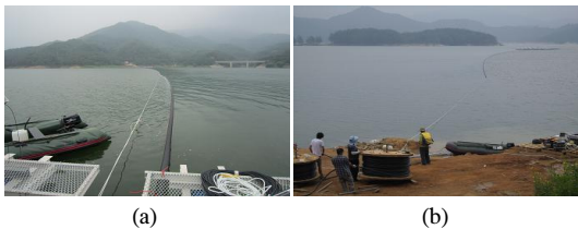
[Fig. 18] Construction of underwater cable pipe (a) Laying of ELP conduit (b) Installment of water cable
