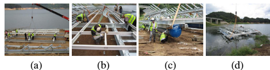
[Fig. 3] Steel structure assembly and launch into water (a) Horizontal and vertical beam assembly (b) Foothold assembly (c) Buoyancy structure assembly (d) Launch into water
