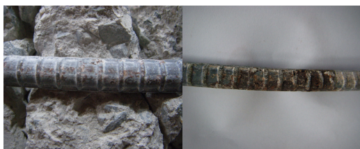
[Fig. 3] Status of steel corrosion after 5 and 10 months
