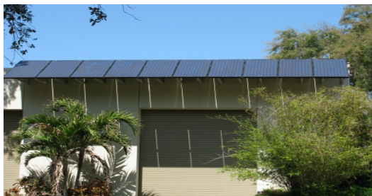
[Fig. 1] PV panels installed in USF campus
